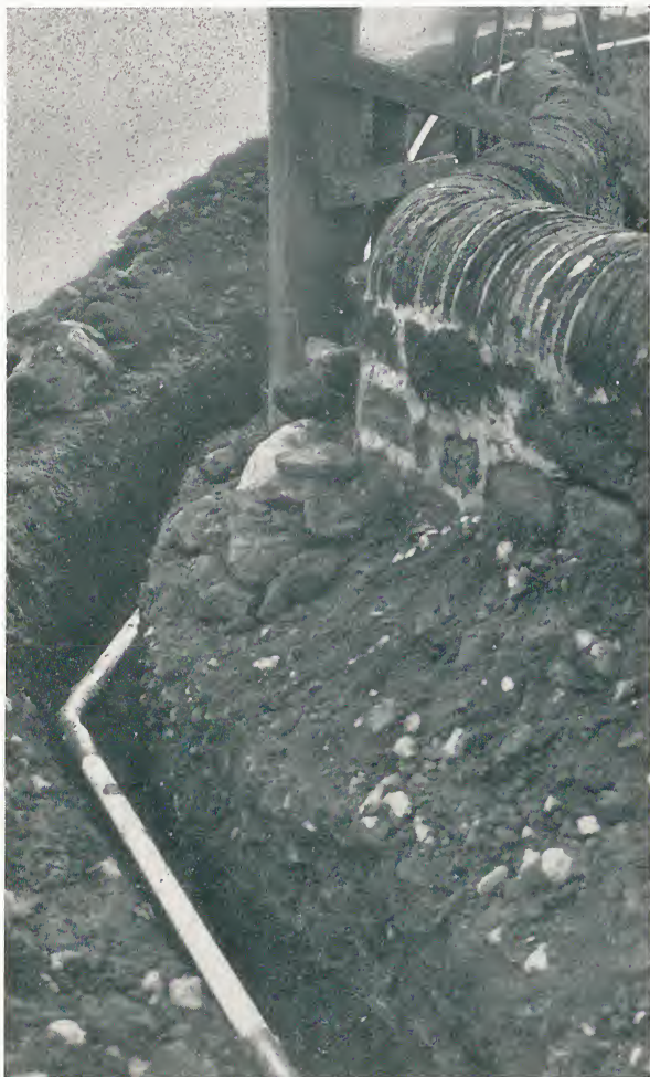
Laying small bore 'S & L' screwed and socketed steel tubes, bitumen lined and 'Security' wrapped, to carry farm water supplies.
